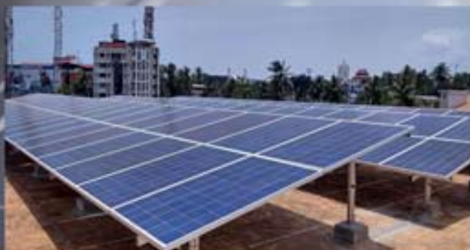
30 kWp Grid Tie project at Reserve Bank of India, TVM
